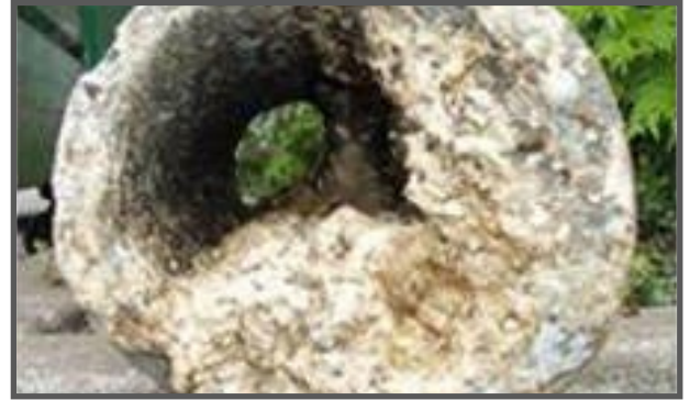
Grease and wipes build-up
