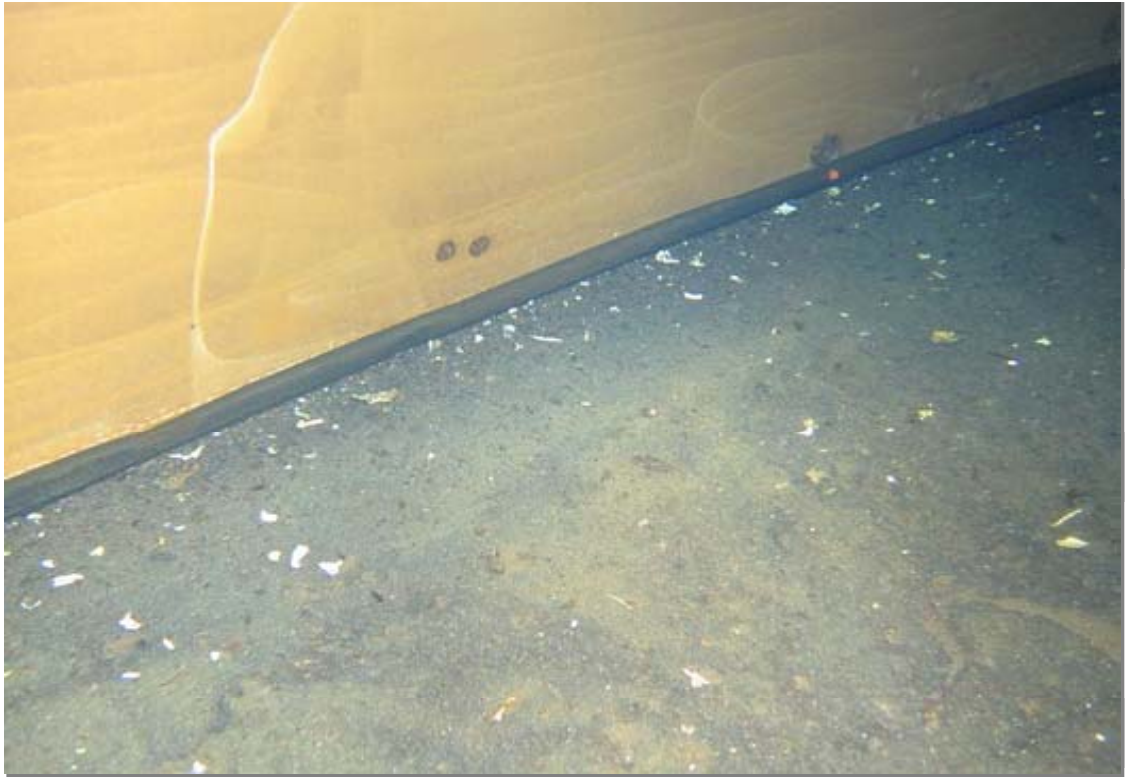
Lower shell and tank bottom. Coatings are in fair condition overall in this zone.
