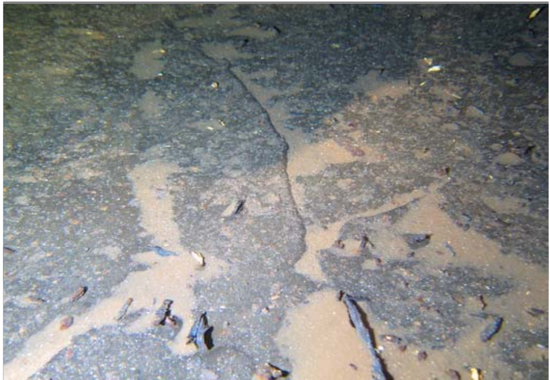
This additional view of the bottom shows some of the corrosion product from the rusting roof rafters above.
