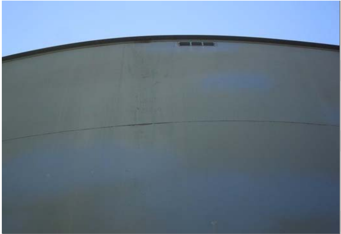
This view represents the typical conditions on the upper shell and shell to roof joint. The upper shell is in good condition with only minor corrosion points noted.
