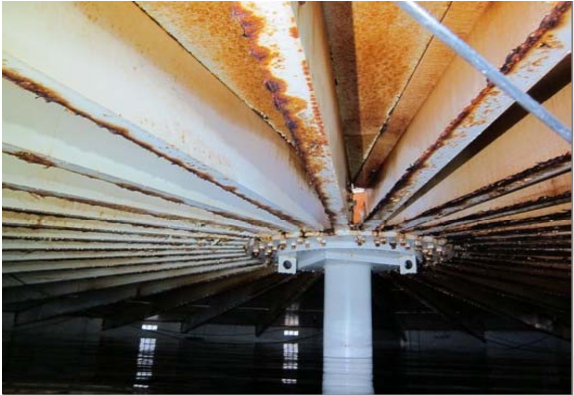
Upper center column, rafters and roof plate. Significant corrosion and associated metal loss are present.
