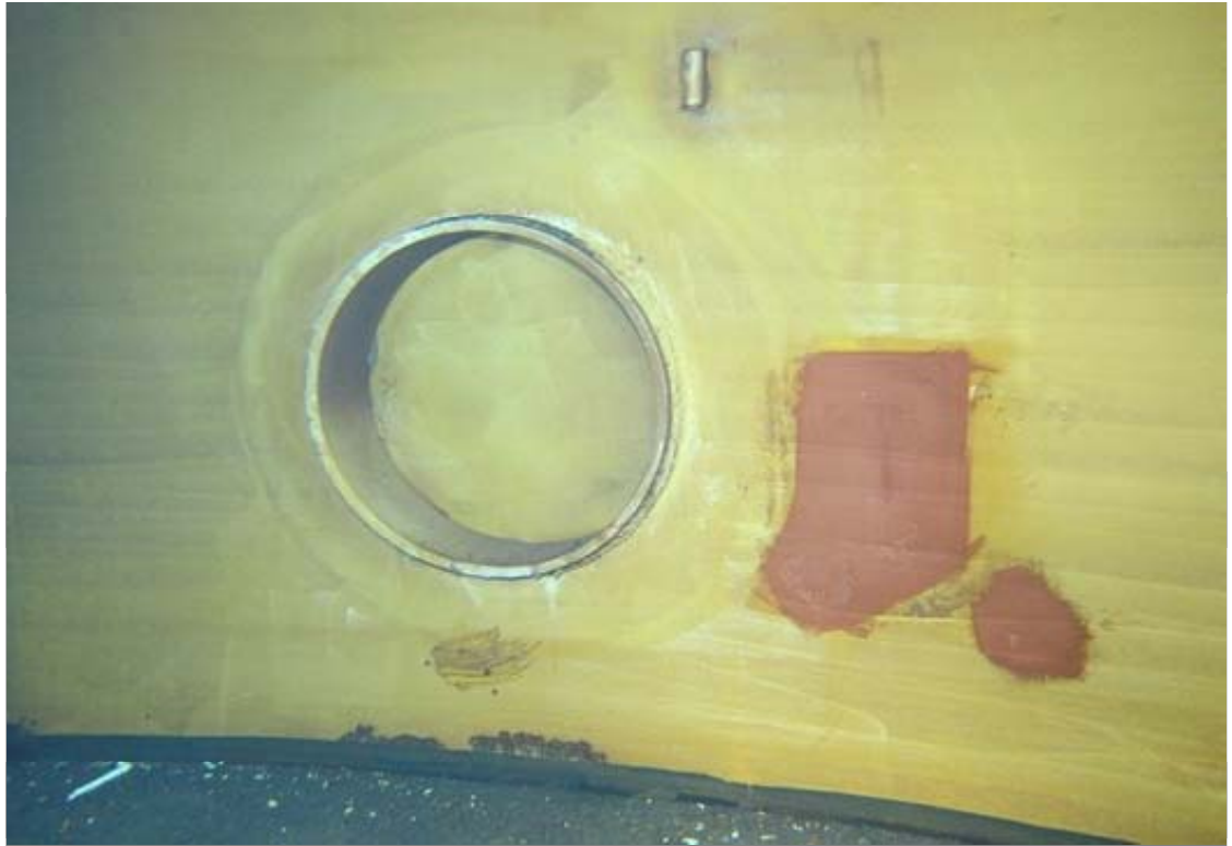
Interior view of the shell manway near quadrant 3. A spot repair is visible to the right and some significant corrosion is present below the manway.
