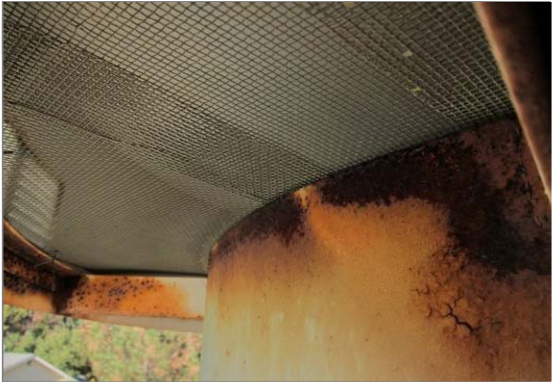
This view of the underside of the vent hood shows that the screen is in good condition. Corrosion is present on the riser but the screen appeared to be bug proof.
