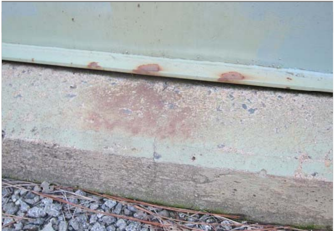
This view of the concrete footing and lower shell shows the typical condition found.
