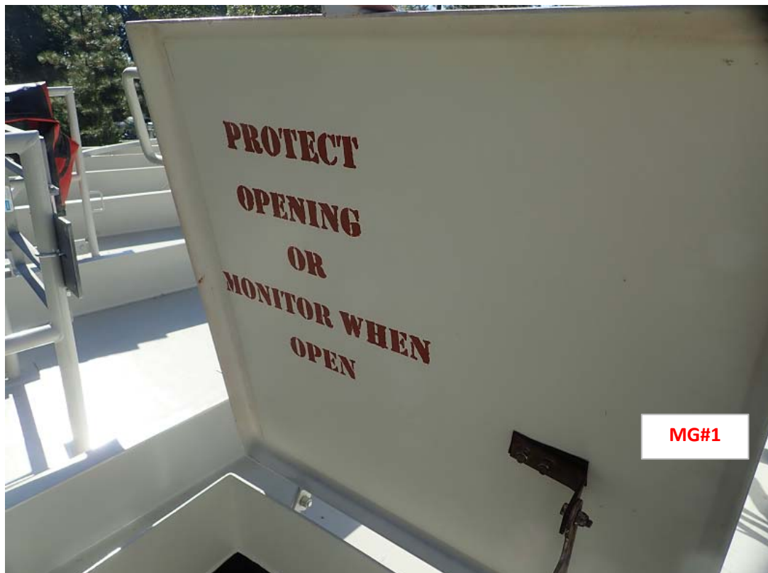
Signage required on new roof hatch.
