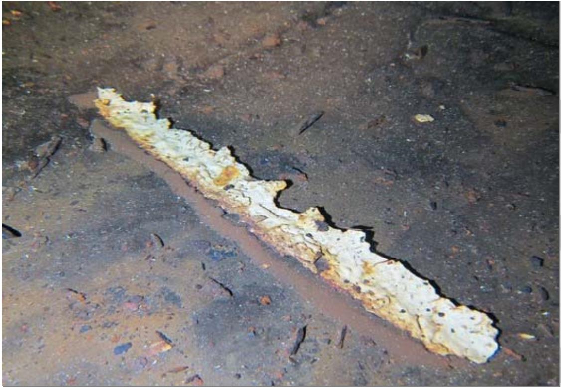
Additional view of interior bottom with coating chip from a roof rafter.
