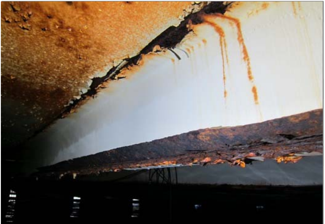
A typical rafter with serious metal loss due to corrosion on the flanges.
