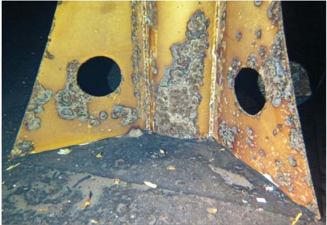
This view shows the column base plate and adjacent bottom plate. Coatings are in poor condition overall on the column and base plate.
