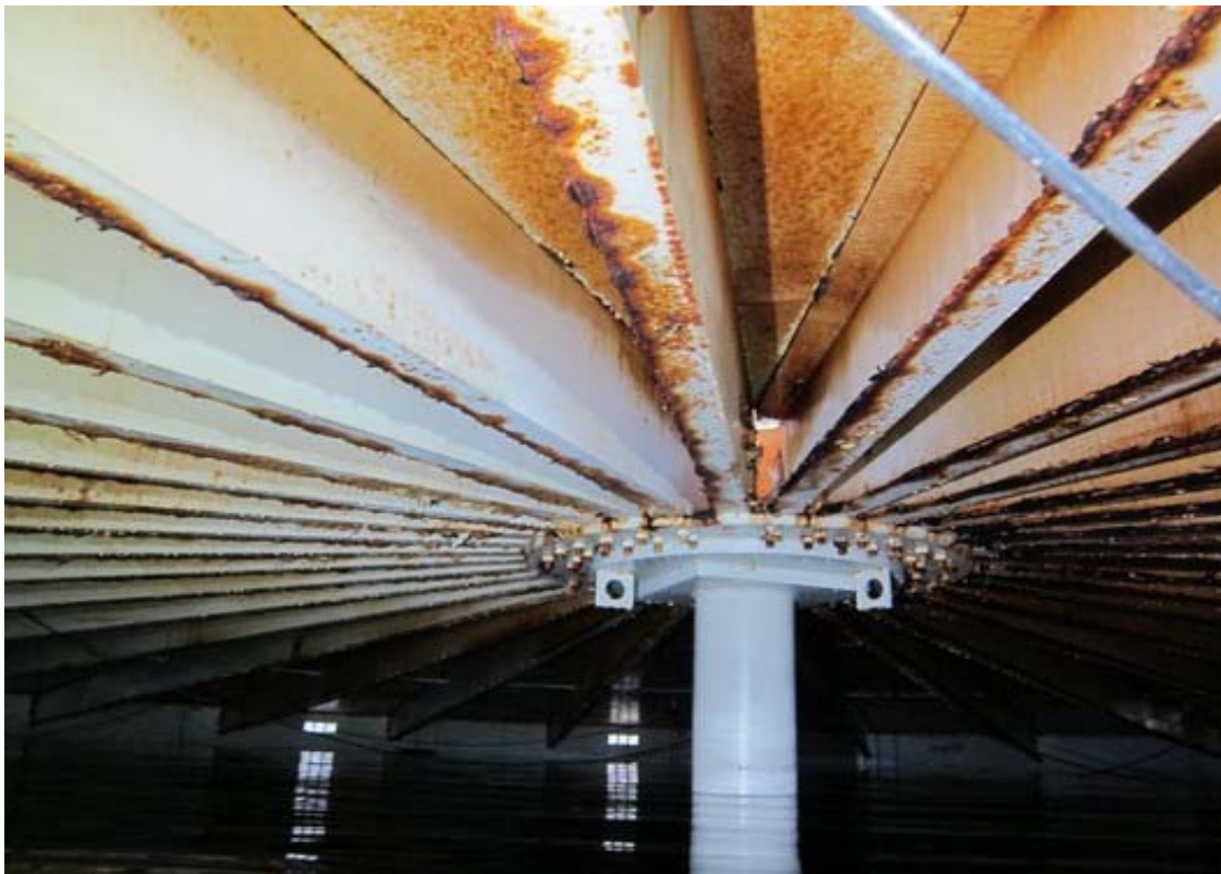
MG #2 existing roof plate, interior center support and rafters to be replaced.
