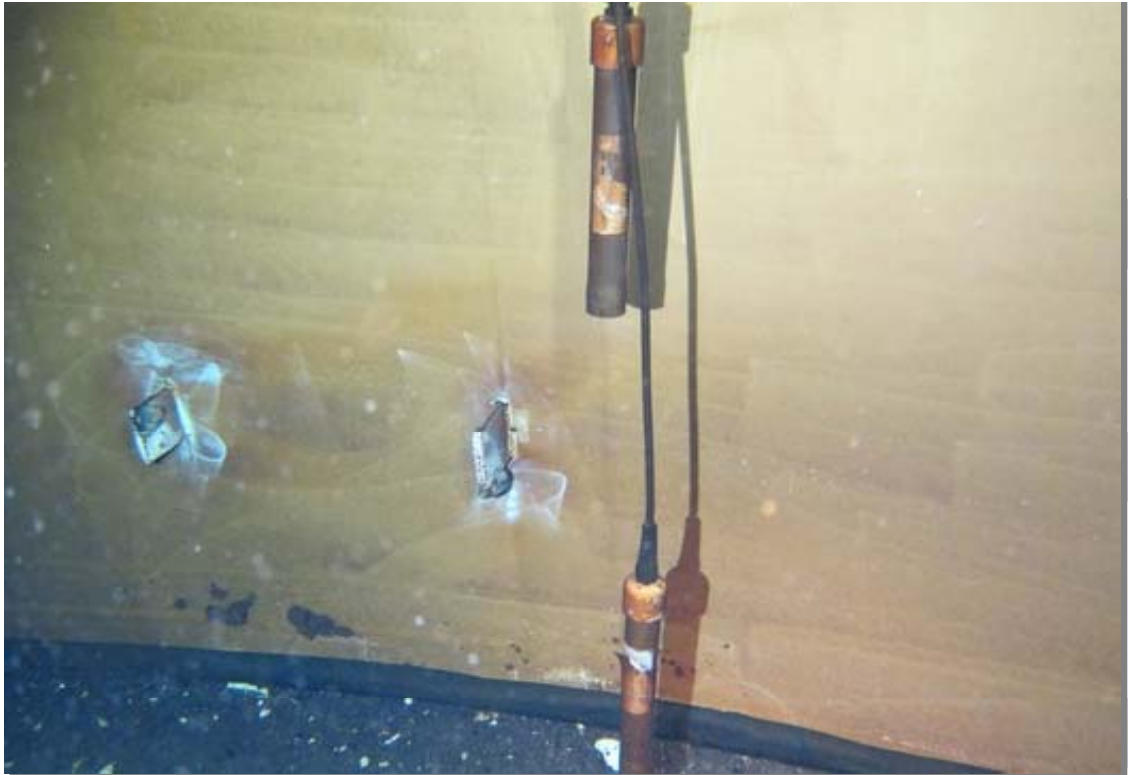
These cathodic protection system reference cells are located below the roof hatch.
