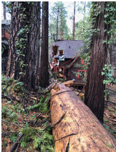
Storm damage in Twain Harte
