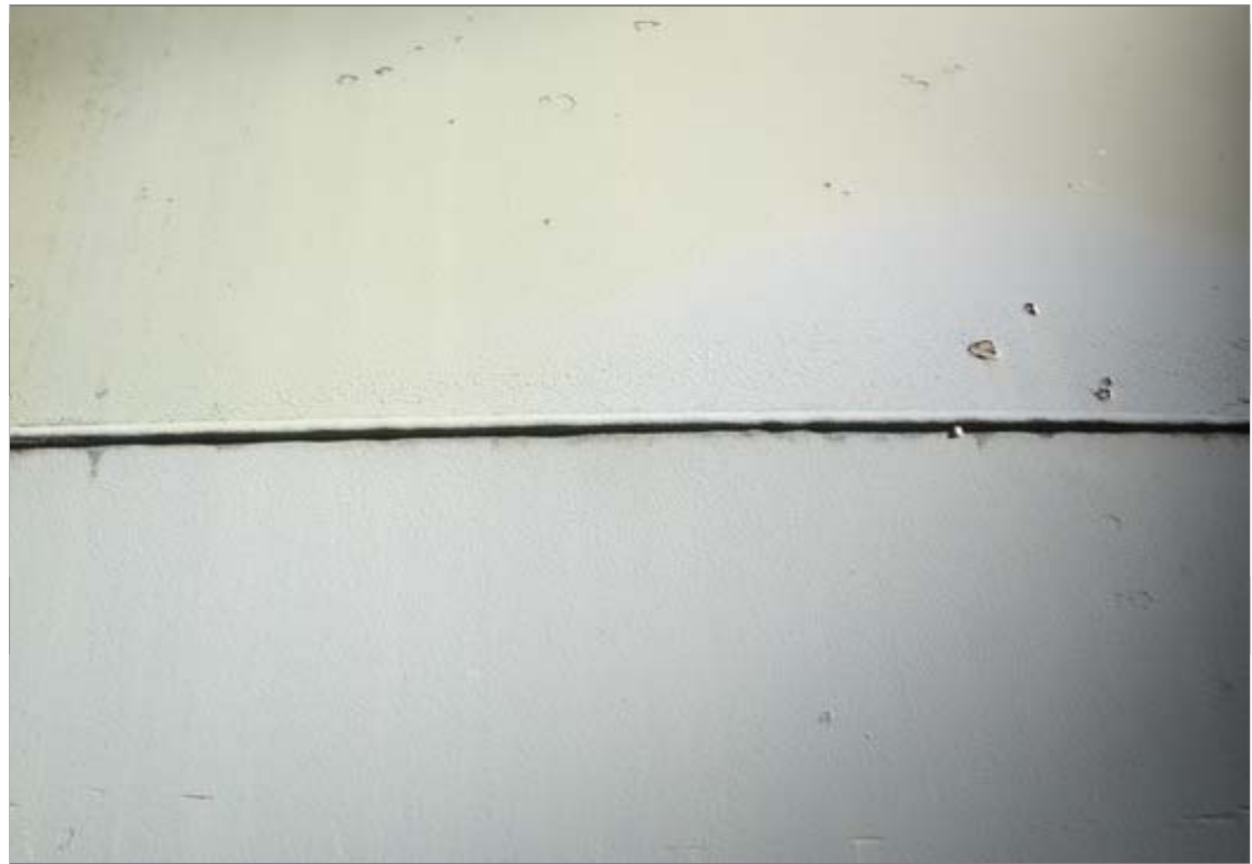
Welds on the exterior shell are generally smoother than the older tank #1 because the welds on this tank are mostly by a mechanized system. Some scattered spatter is present particularly in the areas of welded repairs completed manually.
