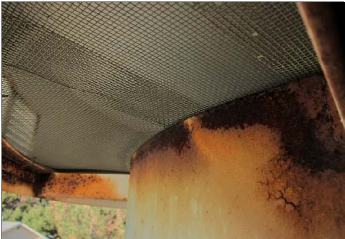
This view of the underside of the vent hood shows that the screen is in good condition. Corrosion is present on the riser but the screen appeared to be bug proof.
