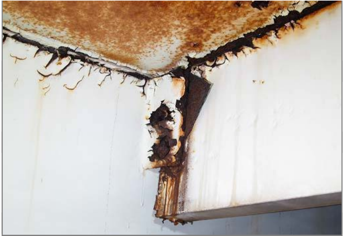
Upper shell, rafter and adjacent roof. Coatings are peeling and general corrosion is present on many surfaces.
