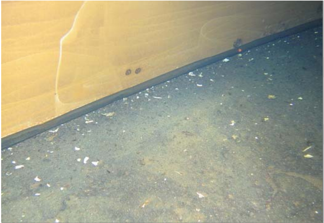
Lower shell and tank bottom. Coatings are in fair condition overall in this zone.
