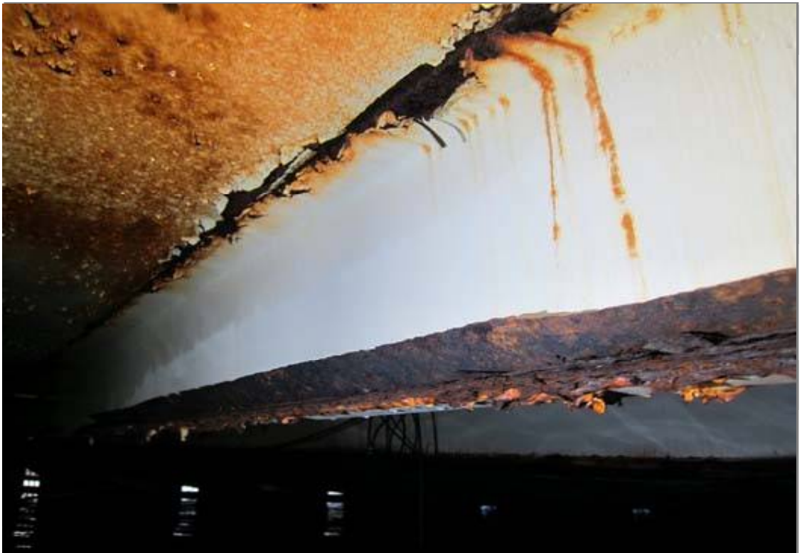
A typical rafter with serious metal loss due to corrosion on the flanges.
