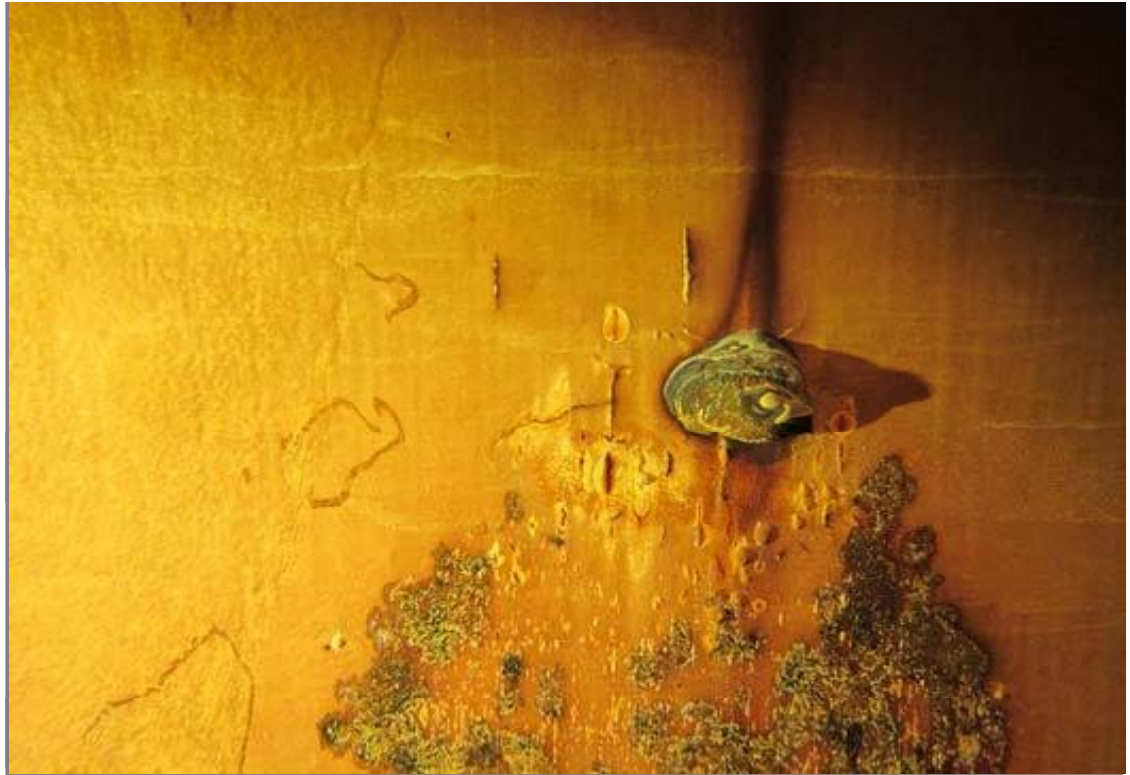
Interior shell in the submersion zone near the manway in quadrant 1. The coatings are cracking and corrosion is present.
