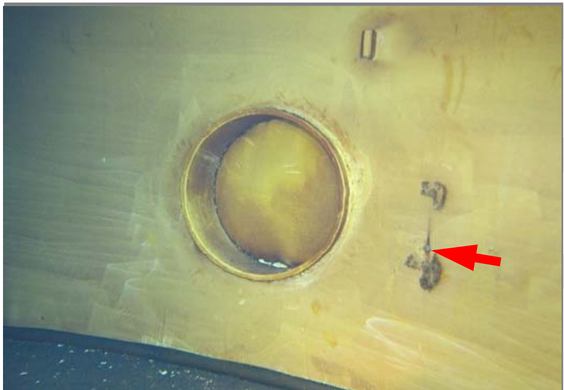
Shell manway in quadrant 1 as viewed from the interior. The spots shown at the right are areas of significant corrosion with a 3/4" diameter nodule at the arrow.
