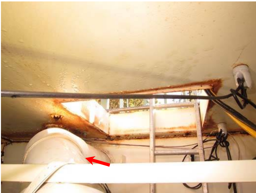
Existing PVC in high inlet pipe on MG#2 that will require protection during work and support from the new roof.
