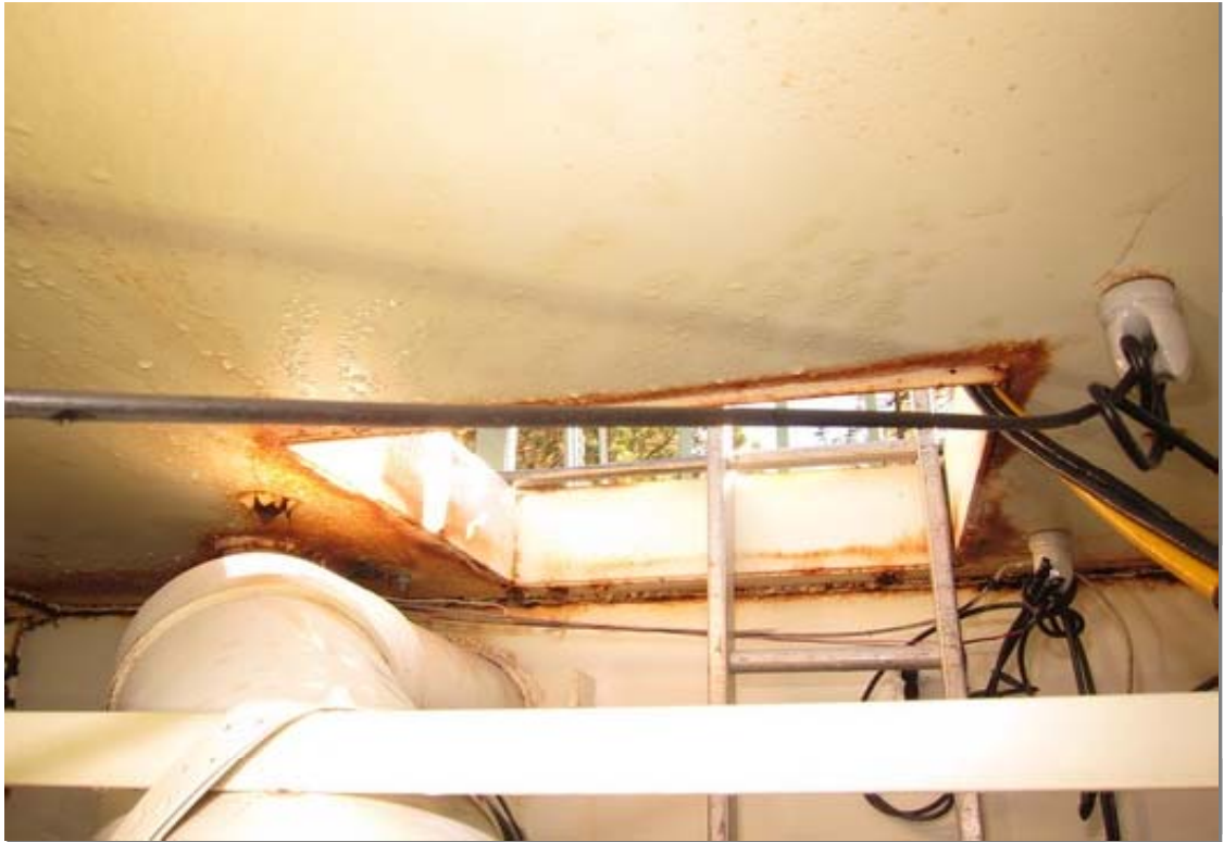
View of the roof hatch from the interior. The diver's entry ladder is visible.
