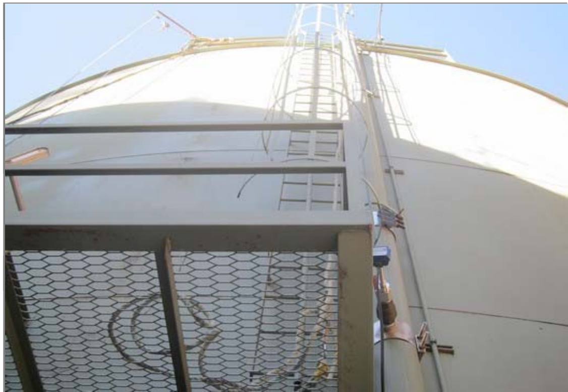
This view from the ground shows the platform, exterior ladder and cage. No significant corrosion is present. The climber safety rail has been painted.
