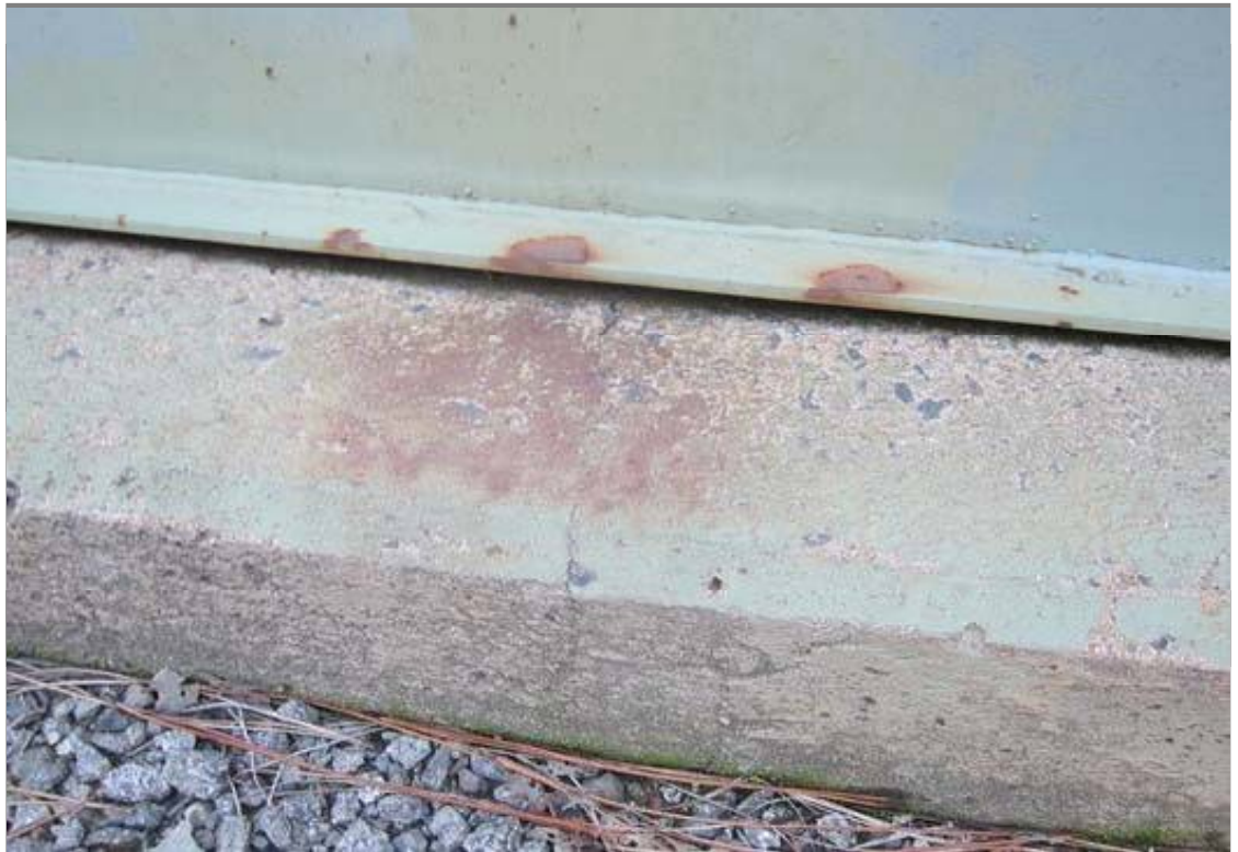
This view of the concrete footing and lower shell shows the typical condition found.
