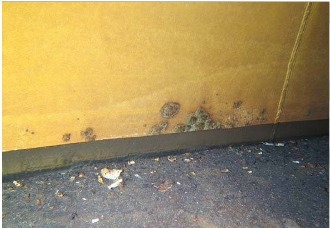
This photo shows an area of the lower shell where coatings are failing. This is an example of the worst condition in this zone.
