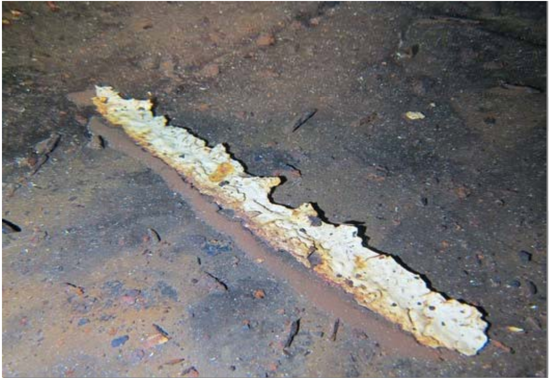
Additional view of interior bottom with coating chip from a roof rafter.
