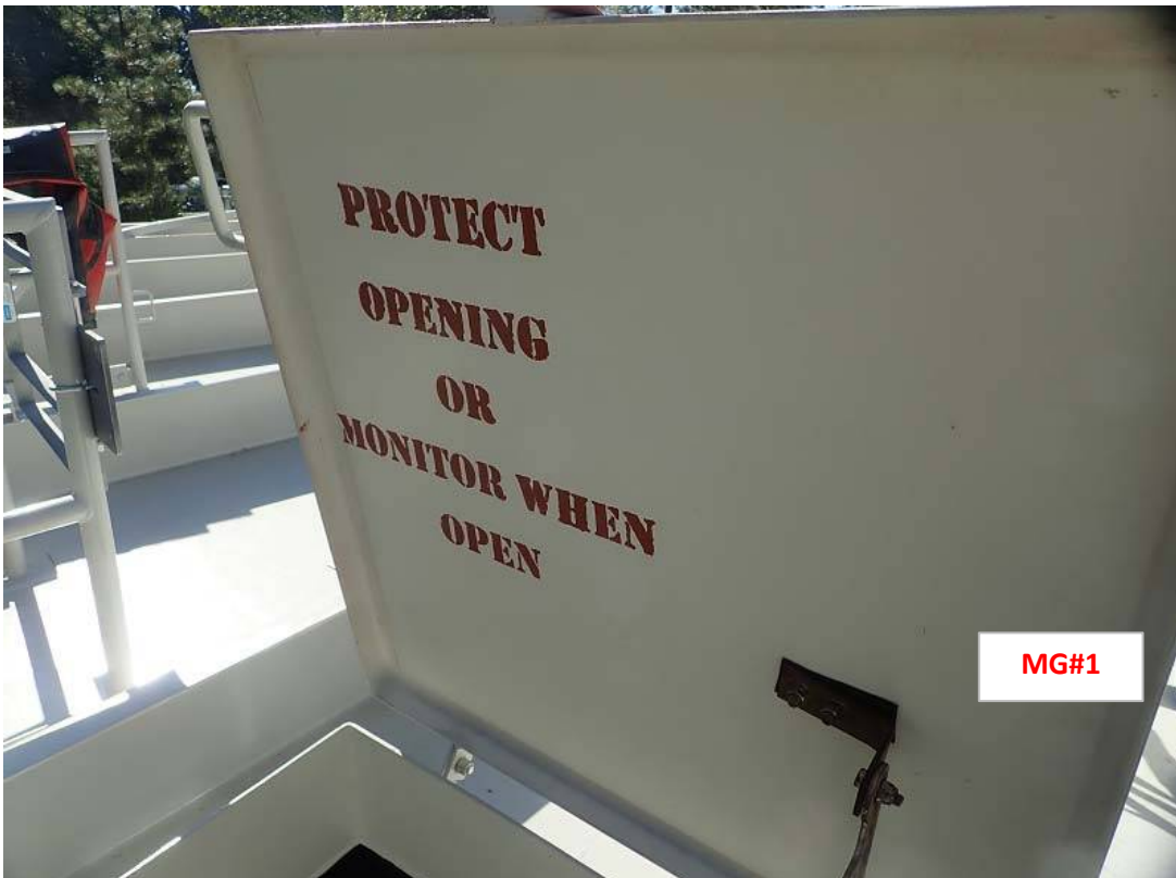
Signage required on new roof hatch.
