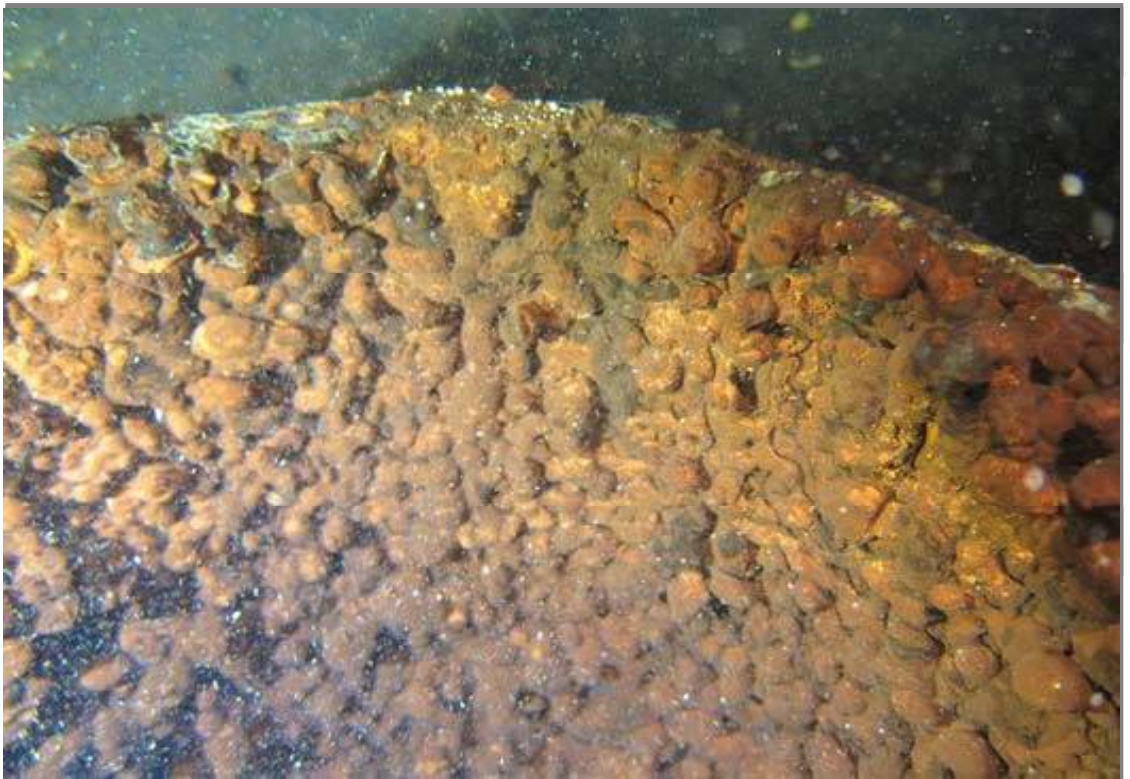
Corrosion nodules on the interior of the outlet pipe.
