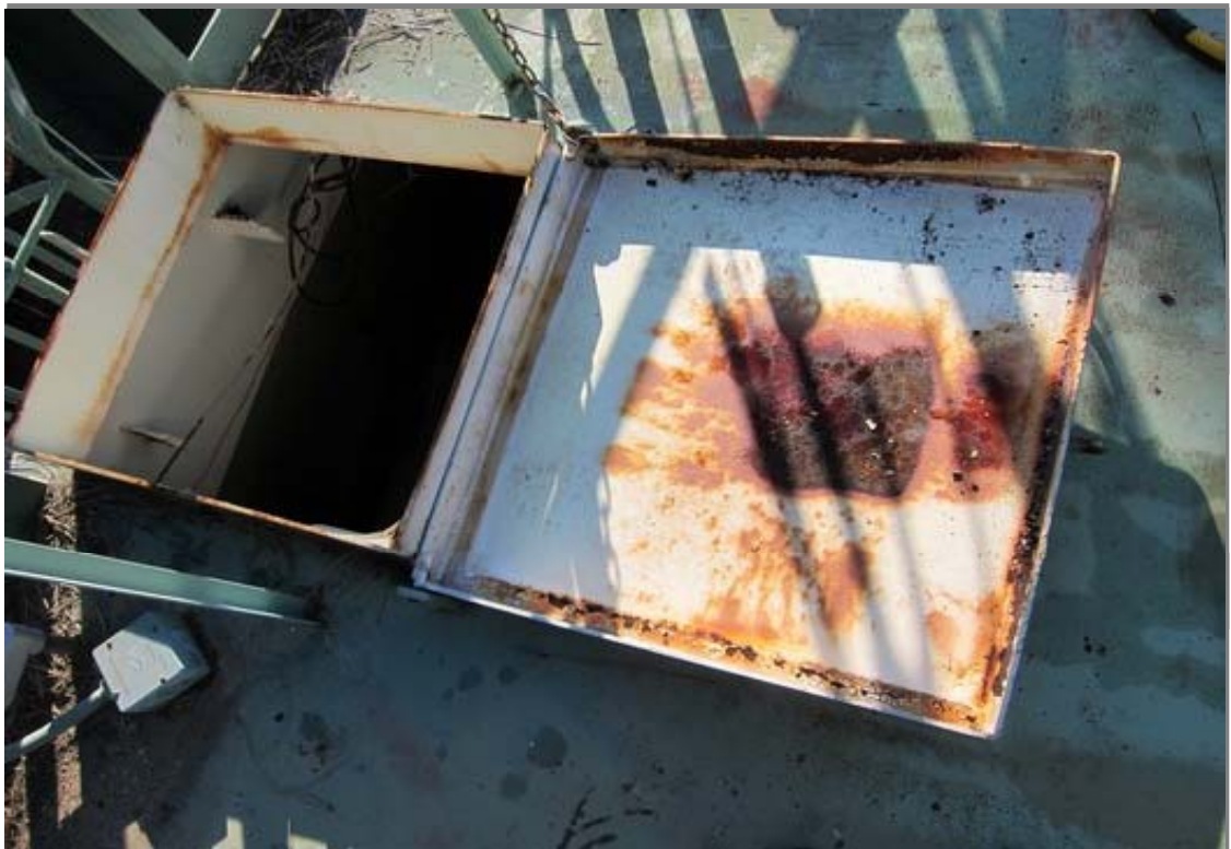
Corrosion on the interior side of the roof hatch.
