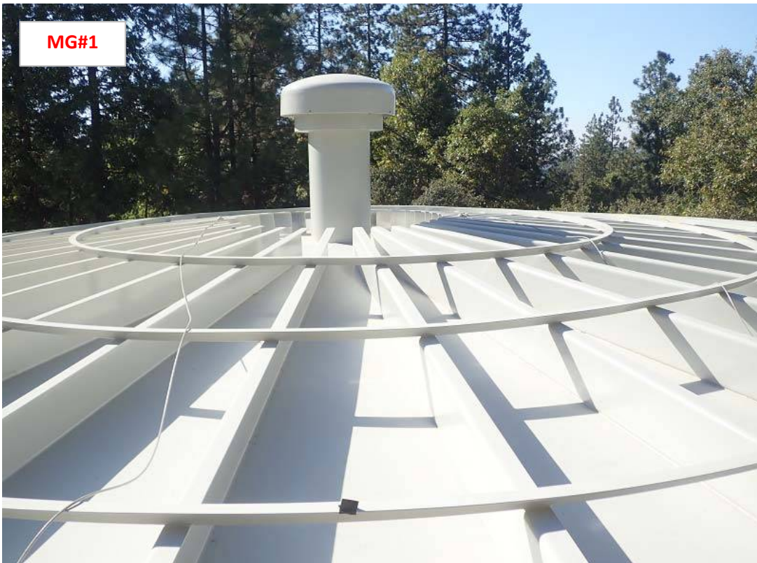
View of exterior roof of previously rehabilitated MG#1. The new roof, vent and guardrail on this MG#2 Rehabilitation project is to be similar.
