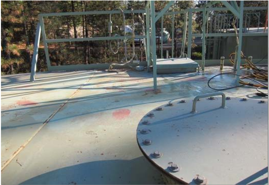
The photo above shows the roof hatch area with guardrail. A second hatch is visible in the foreground.
