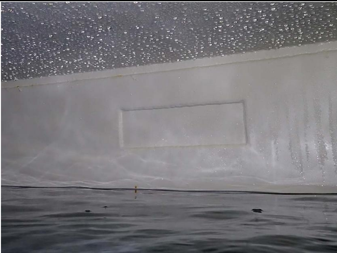
View of acceptable shell vent closure.
