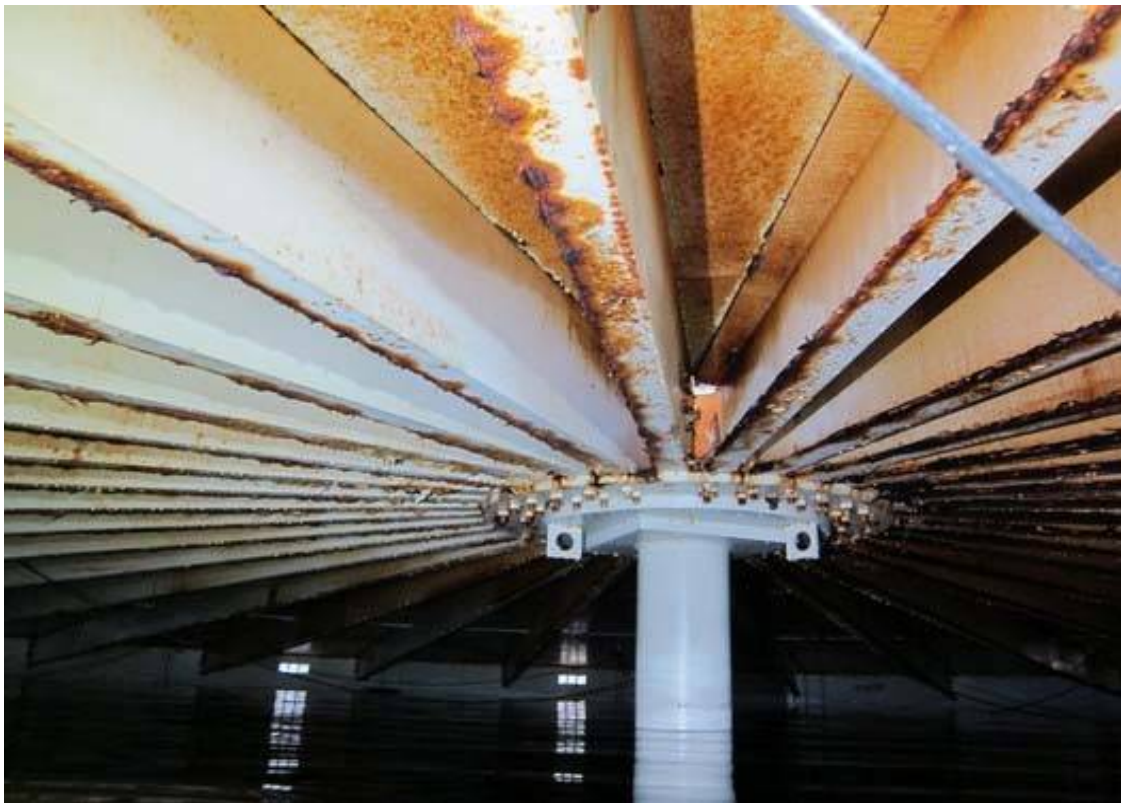
MG #2 existing roof plate, interior center support and rafters to be replaced.
