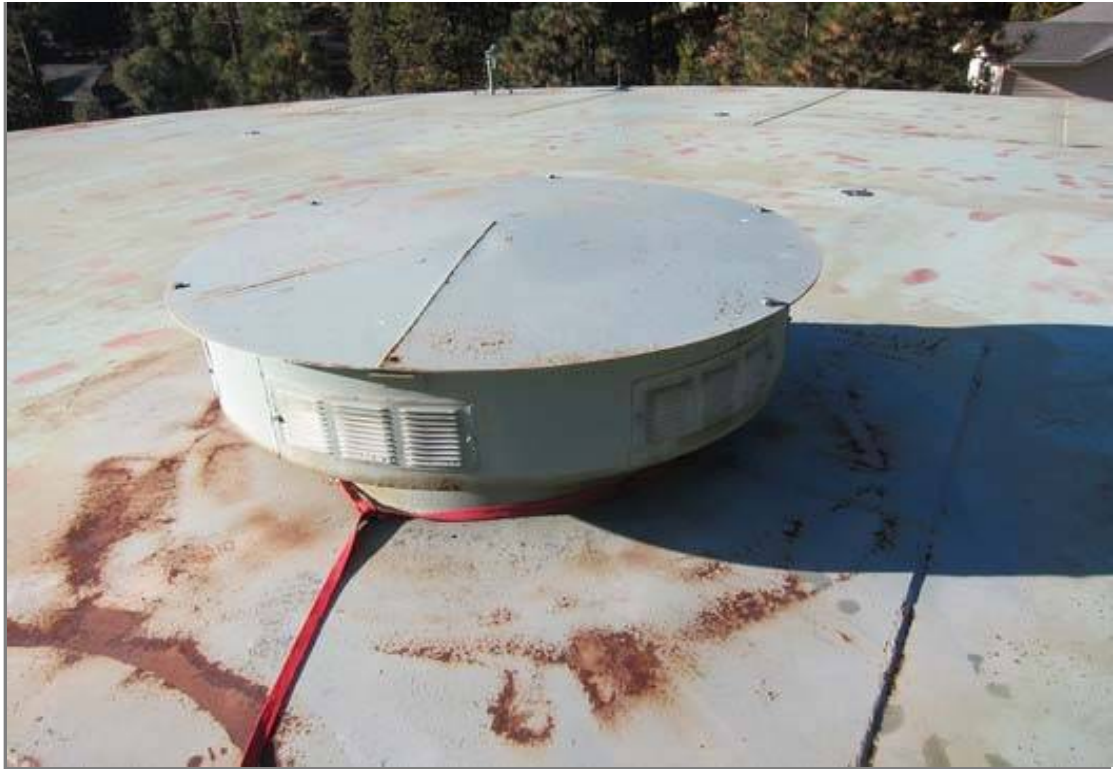
The roof vent consists of a steel cover over a steel riser pipe.
