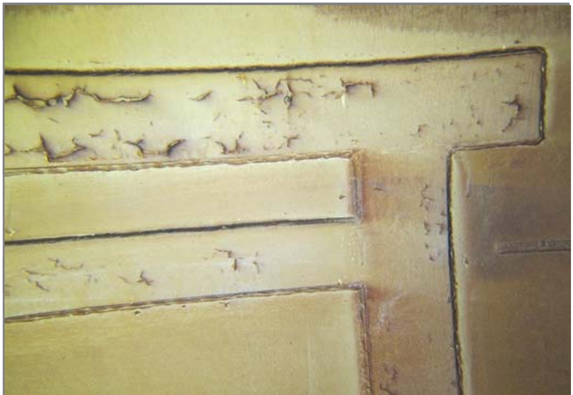
This view of cracked coatings is where a shell opening (door sheet) was cut and re-welded upon completion of the work. This area has a particularly high concentration of coating failures.
