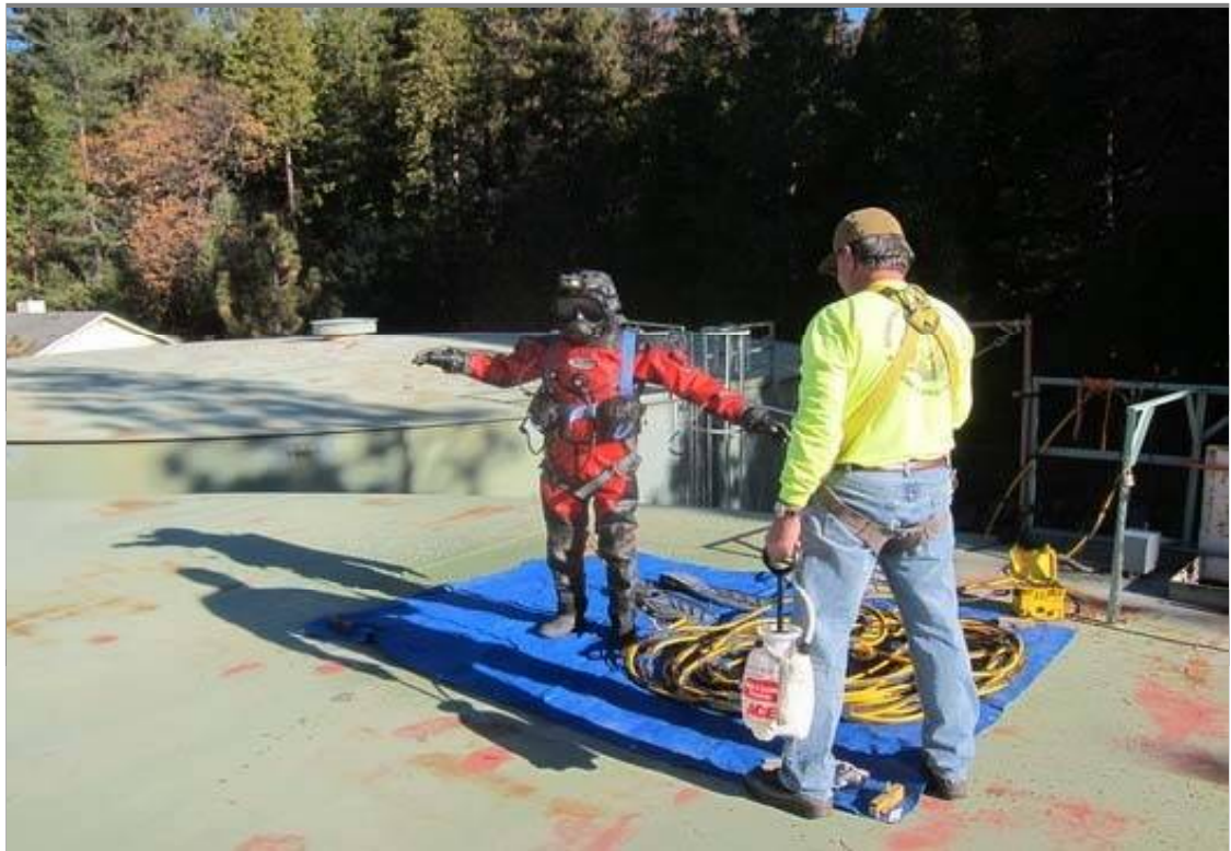
Diver and equipment are disinfected with the chlorine solution just prior to entry. This procedure is pursuant to AWWA disinfection standards for potable water diving.
