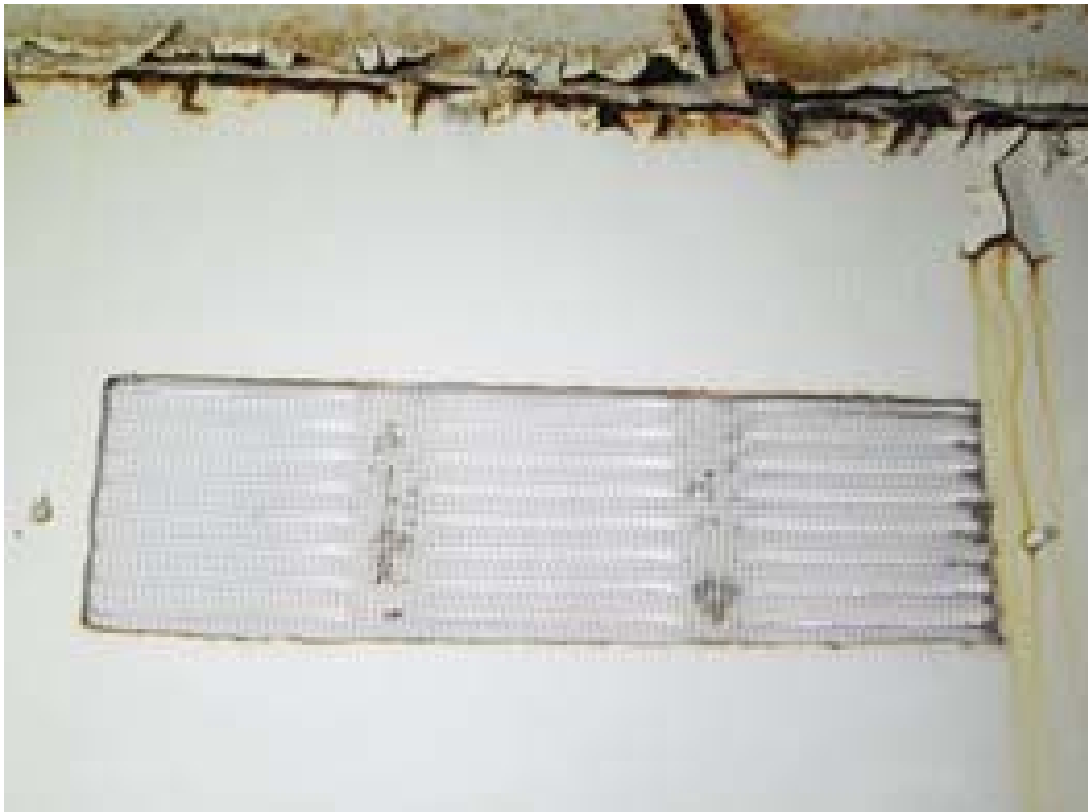
View of typical existing shell vent. Cover plates are to be installed as part of the Work.
