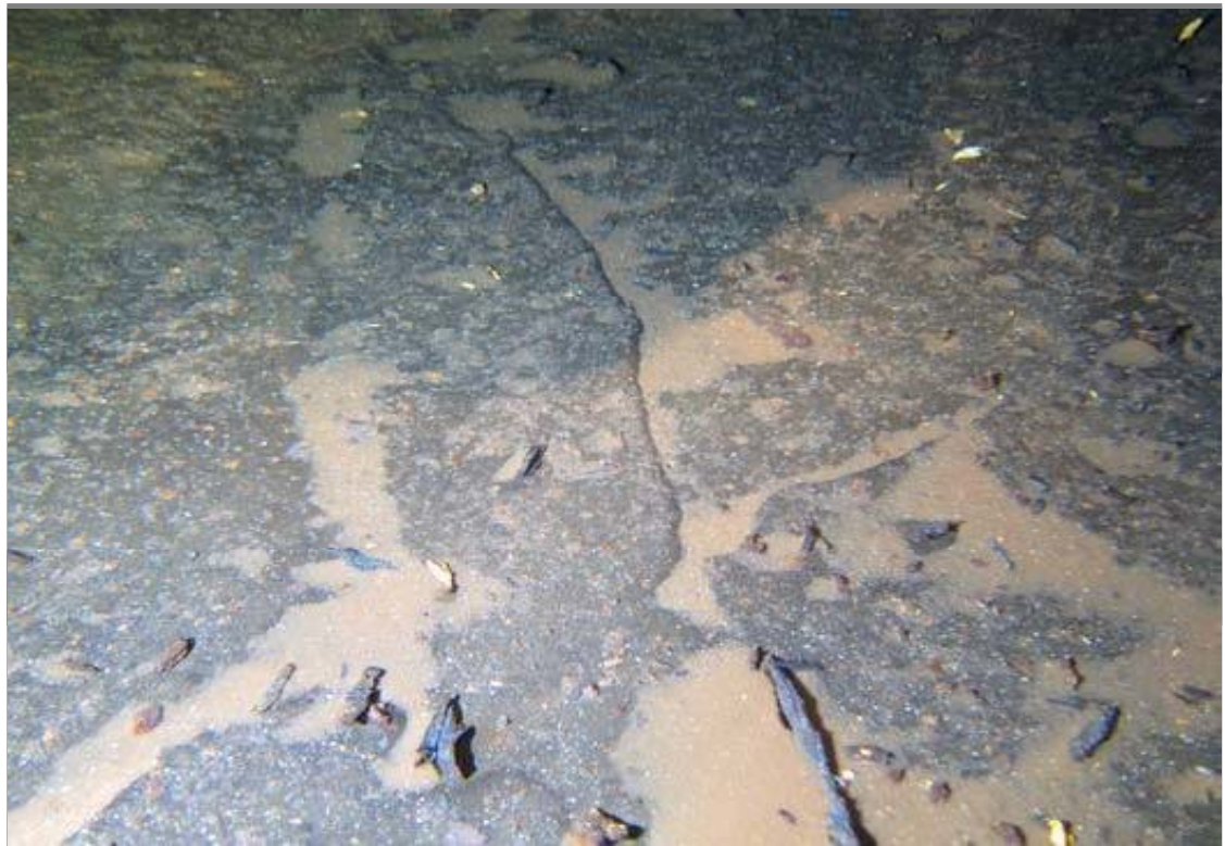
This additional view of the bottom shows some of the corrosion product from the rusting roof rafters above.
