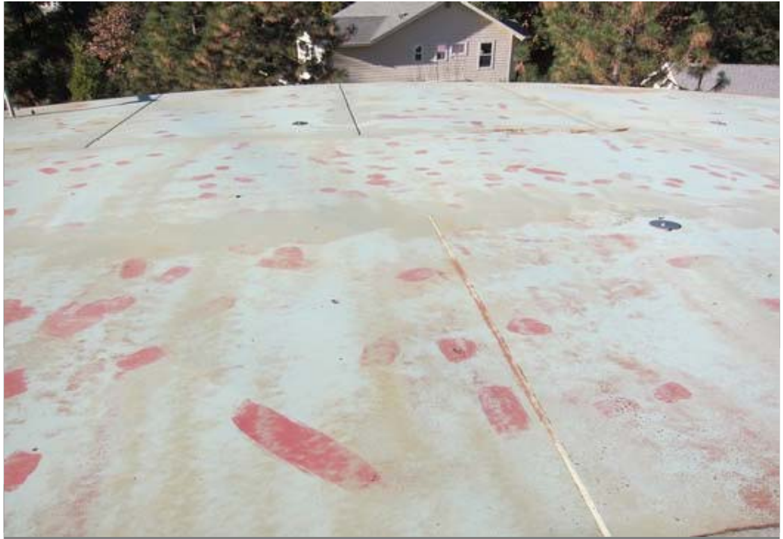
This view indicates the overall condition of the roof. The roof plate (steel) is in good condition but coatings are in poor condition.
