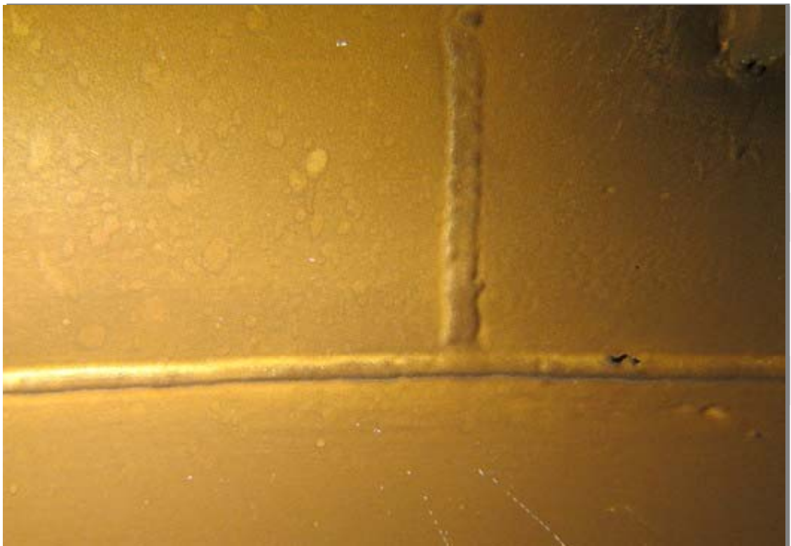
Interior shell in the submersion zone. This view shows a junction between a horizontal and vertical shell joint. The interior shell steel appears to be in good condition overall.
