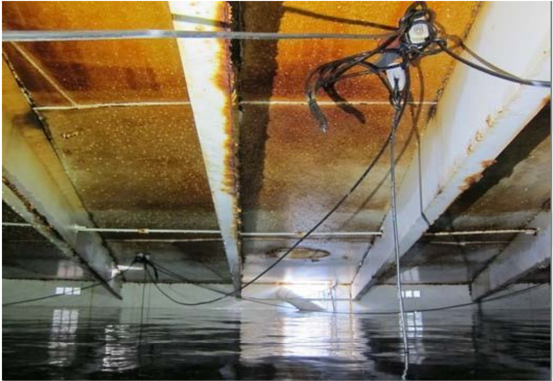
This broad view of the roof is looking toward the roof hatch from near the center.
