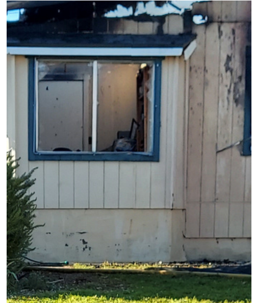
(Above) The closed door, which you can see through the window, spared this room from severe damage
