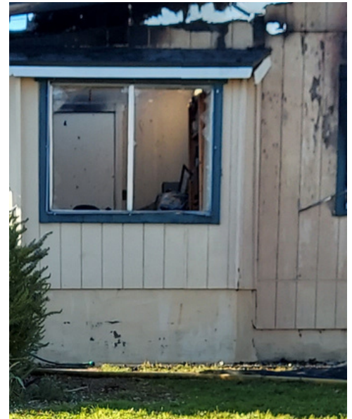
(Above) The closed door, which you can see through the window, spared this room from severe damage
