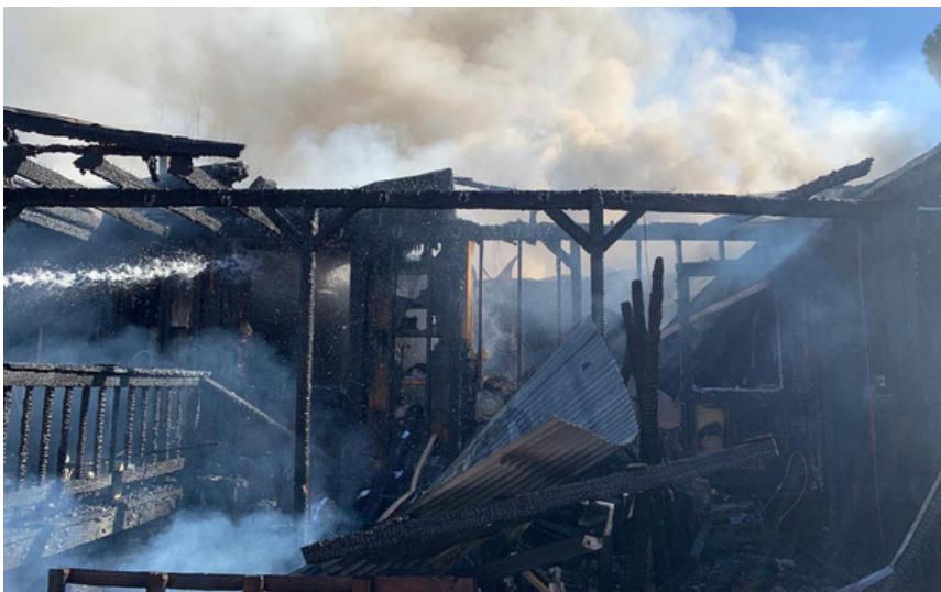
(Left) Unfortunately, the entire house was destroyed, except for the one room that had the door closed
