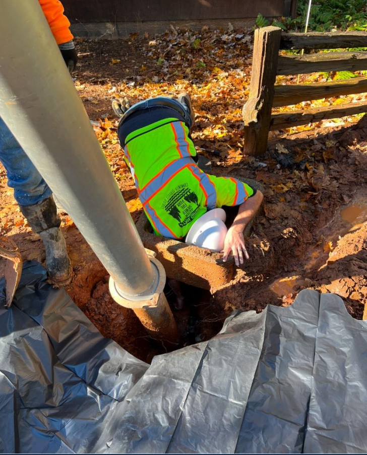
Top Left: Spruce Dr. leak
