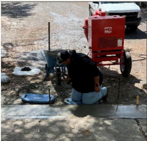
Final concrete work from a leak
