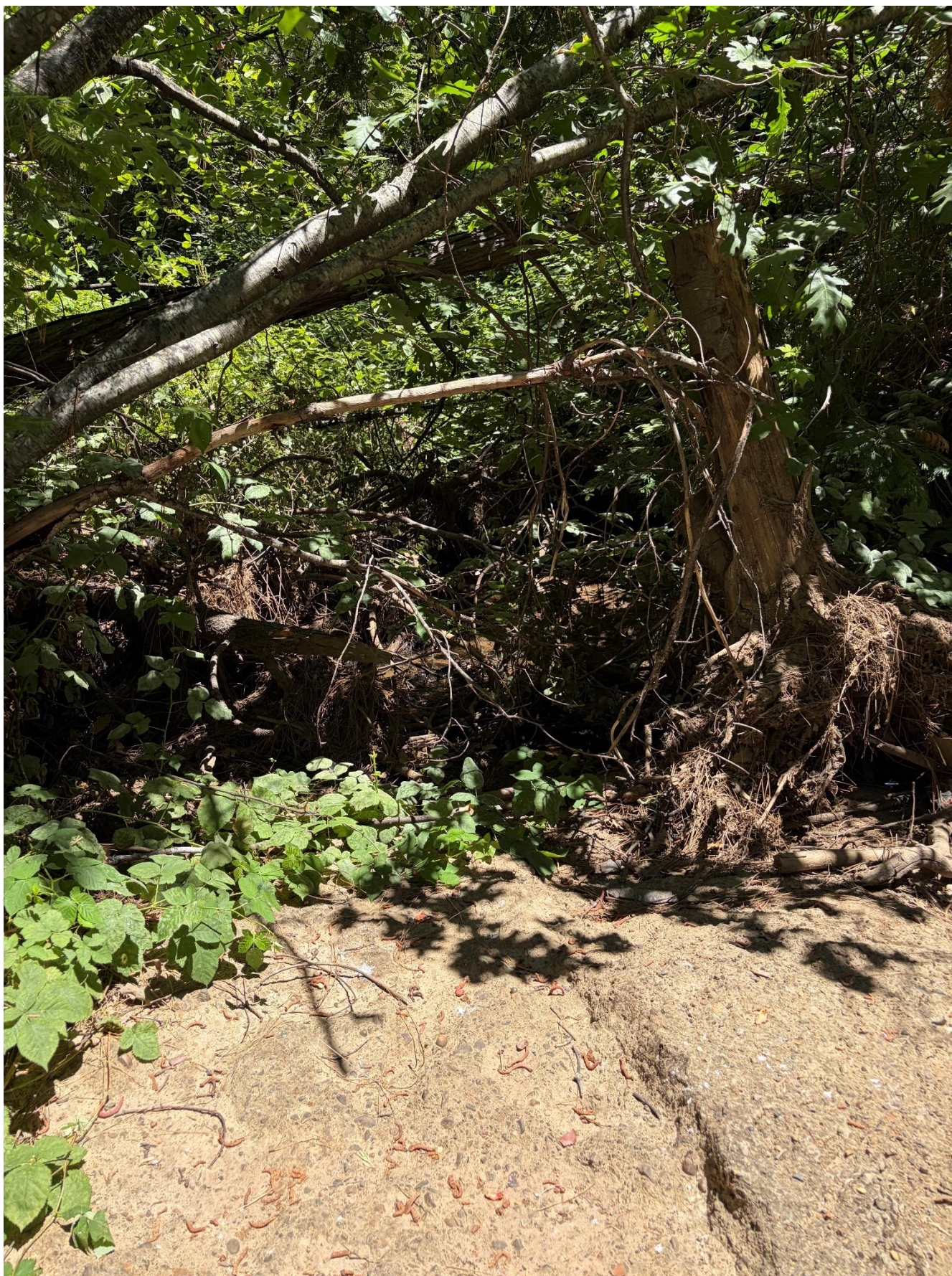
Upstream side of encasement blocked with debris and dense vegetation. Water still flows through pipes, but only water in stream currently is TUD release from ditch to Twain Harte Lake.
