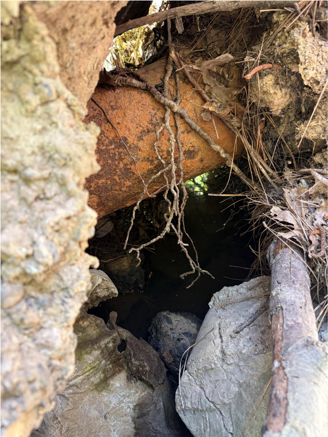
Exposed sewer line at edge of concrete encasement. High storm flows has eroded the bank away and all dirt at the edge of the concrete encasement, creating a potential for failure and sewer overflow into Twain Harte Creek and Twain Harte Lake.
