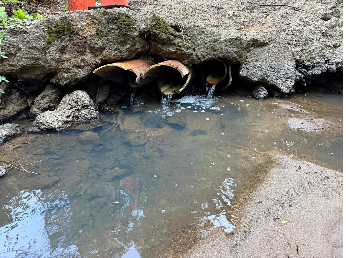
Existing drains (downstream side of encasement) that stream flows through when not high enough to flow over top of encasement. High flows have cause undermining beneath encasement.
